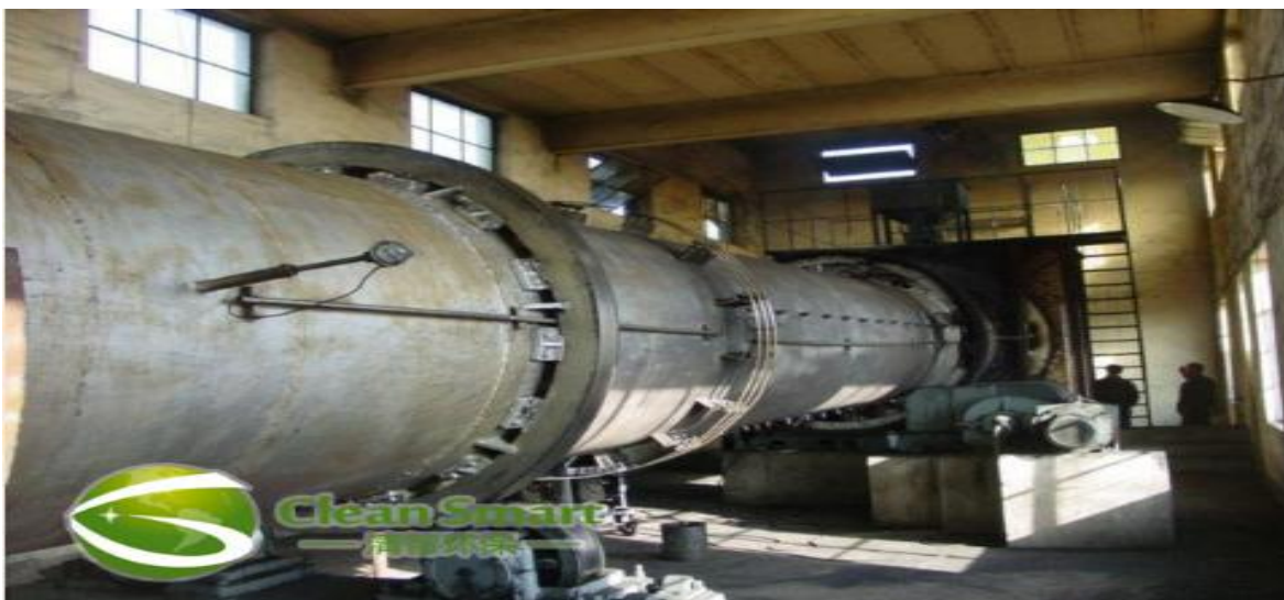
Figure-11: Continuous carbon activation furnace rotary kiln.
